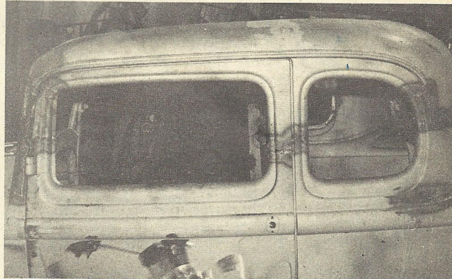
Everything is aligned and welded. Doors and top are now ready for final body work.
